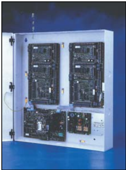
AMAG multiNODE control panels communicate with HID proximity readers and electrified door hardware.
